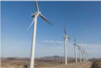
TURKANA WIND FARM
