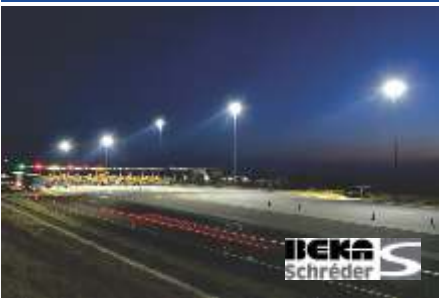
Stadium floodlights, security, parking areas, etc.
